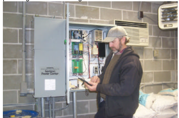
Dallas Rural Water Manager Dana Gann – Viewing The Levels In The Remote Water Towers With The Palmtop Interface
