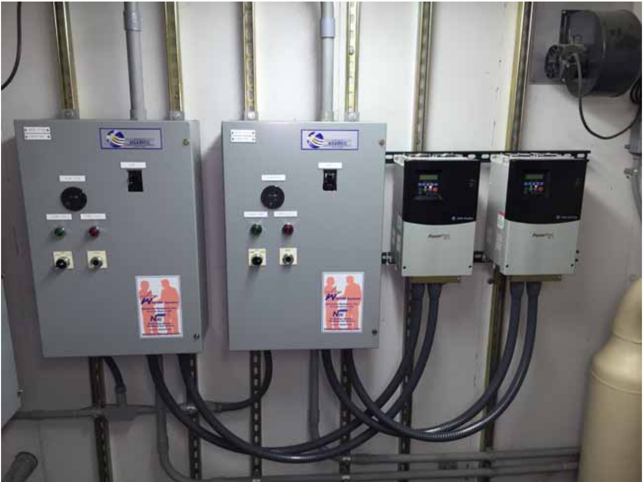
PowerFlex 400 VFDs Installed In A Duplex 25HP Pump Station: Williamsville, IL. These VFDs were installed as a replacement/upgrade to existing Soft Starters. Load Reactors were installed within the Circuit Breaker/Soft Starter Panels (Left).
