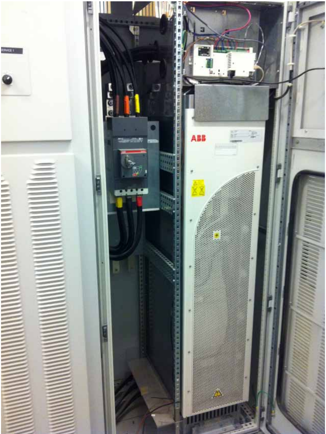
An ABB Model ACH550 VFD. At a Water Plant, Feeding a 250HP High Service Pump.
